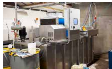
The central filtration system for filtering coolant.
